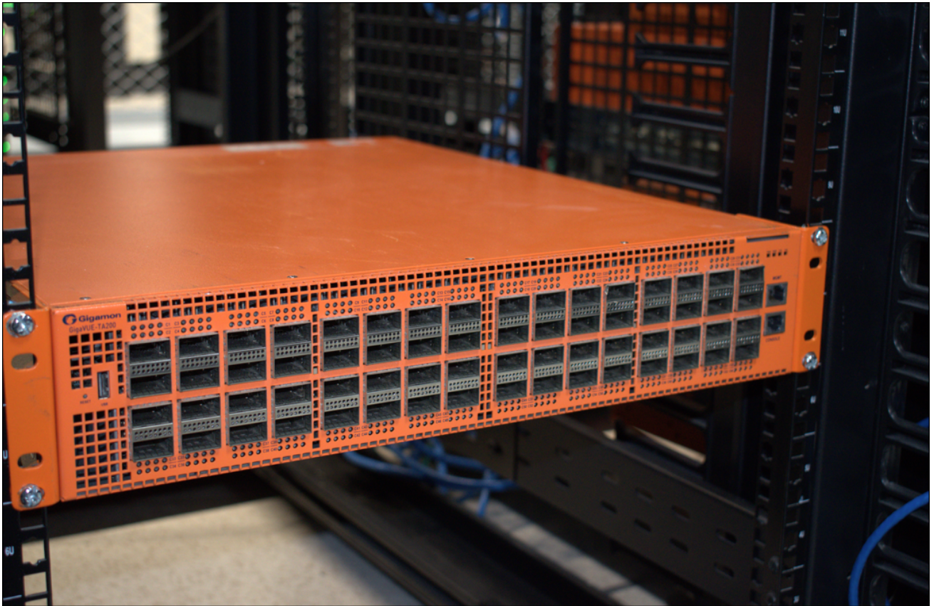
Figure 5 Front View of the Mounted Node to the Four-Post Rack
