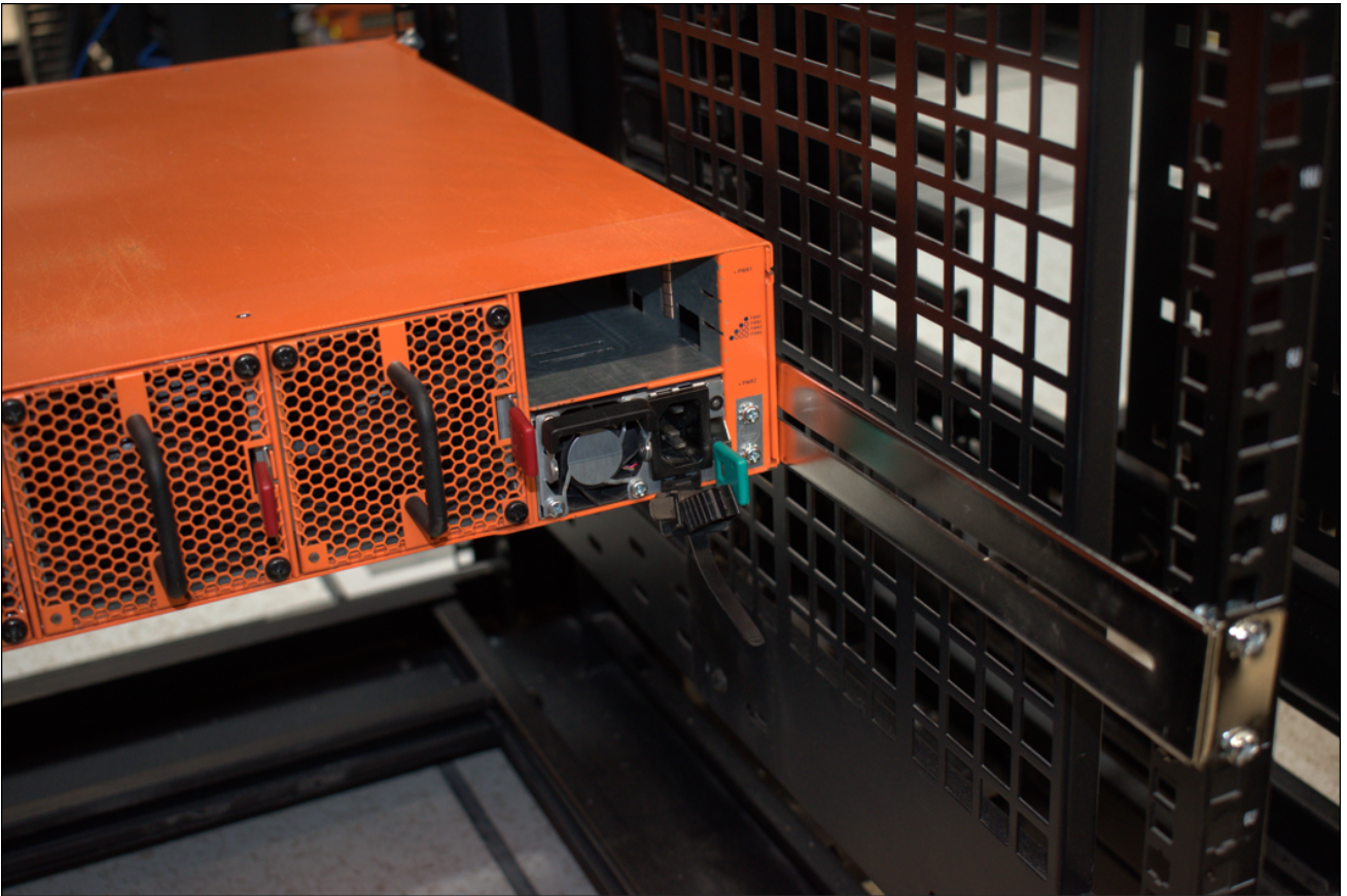
Figure 6 Rear View of the Mounted Node and Rails on the Four-Post Rack
